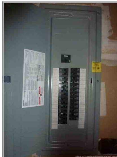
Circuit Breaker Panel; garage
