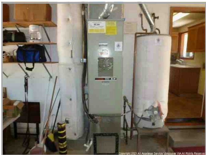
Furnace (gas)/Hot Water (gas) (Location: Two-Car Garage)
